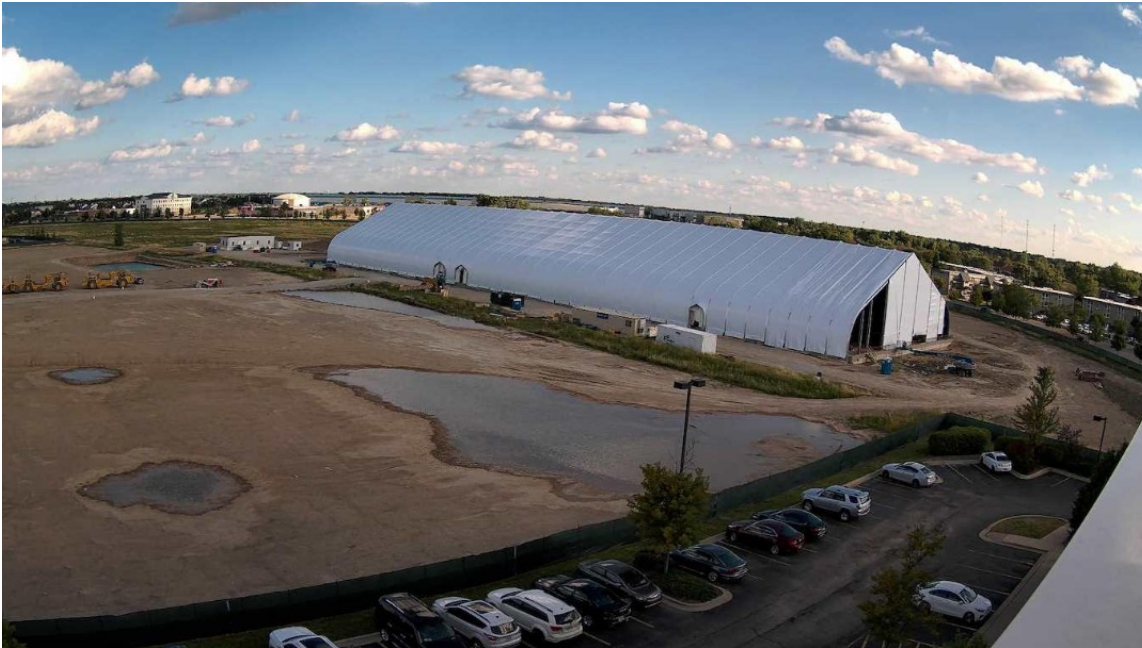
Construction continues at The Temporary by American Place, a new casino anticipated to open in the fourth quarter of 2022 in Waukegan, Illinois.
