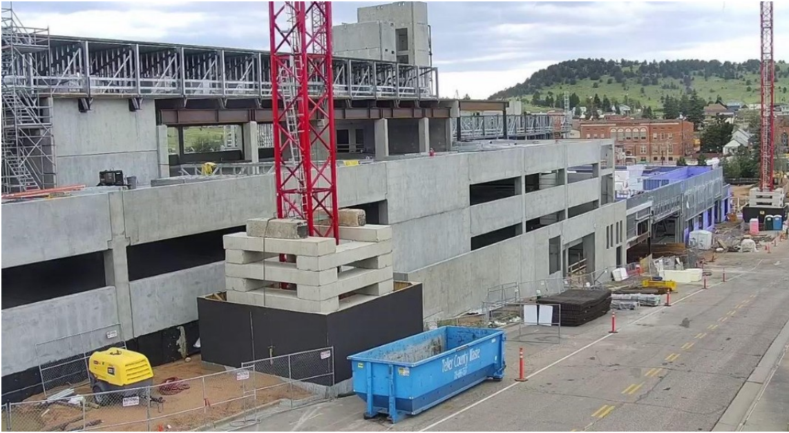
Construction continues at Chamonix Casino Hotel, a new luxury gaming destination anticipated to open in mid-2023 in Cripple Creek, Colorado.
