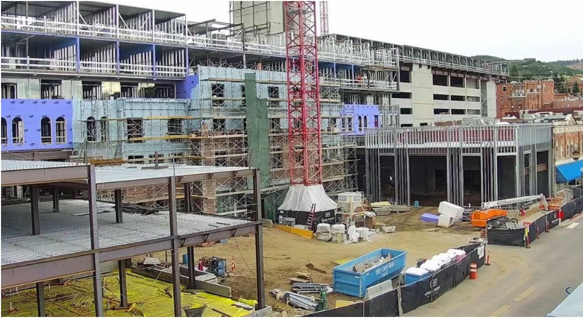
Construction continues at Chamonix Casino Hotel, a new luxury gaming destination anticipated to open in mid-2023 in Cripple Creek, Colorado.
